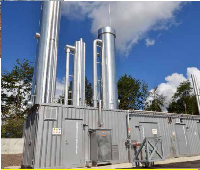
biogas upgrading -water scrubbing (1400 m3 raw biogas/h) .
