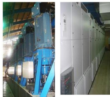
Sugar centrifuges fitted with ABB Motor and VFD at Al Khaleej sugar mills centrifuges
