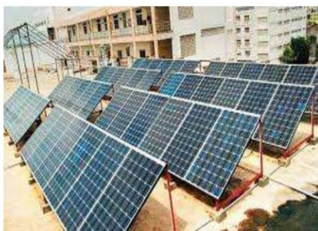
Rooftop solar photovoltaic plant
