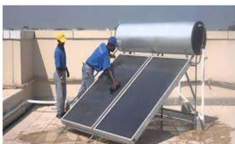
Rooftop solar water heater
