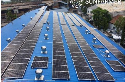
Steel Industries : 163 kWp On-Grid Solar PV System
