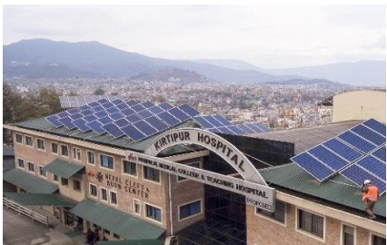
Hospital: 66.8 kWp On- Solar System with Net Metering
