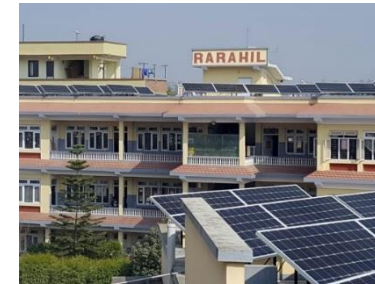
School: 40.2 kWp On-Grid System with net metering
