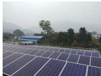
Cable Industries: 165.8 kWp On-Grid solar system
