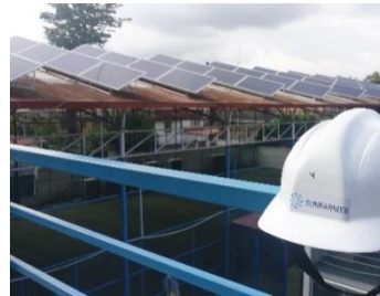
School: 40.96 kWp On-Grid solar system
