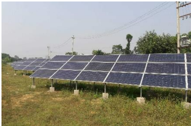
Drinking Water: 100 kWp On-Grid Water Pumping System
