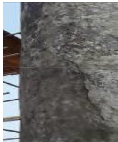
Photo: Leakage cracks in chimney
