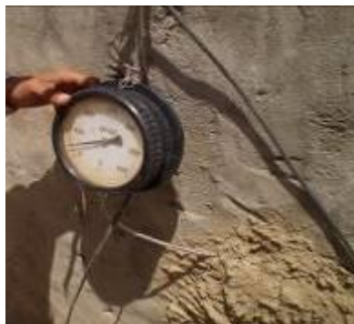
Photo: Temperature gauge installed at chimney
